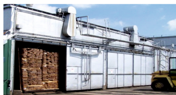
Steam heated drying kiln
