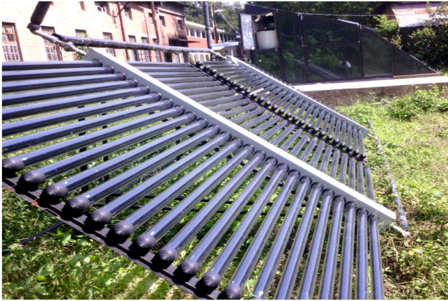
Figure 7: Thermal energy storage system assisted with Evacuated Tube Collector (ETC) array
